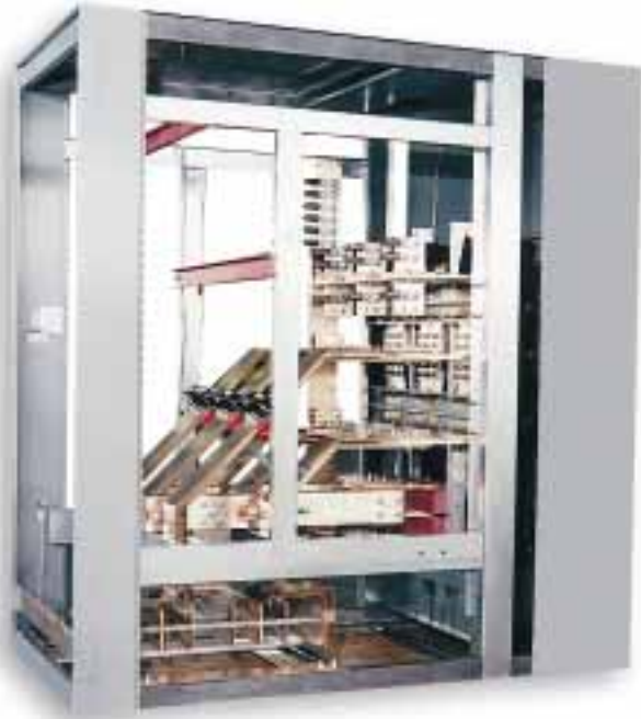
Fig. 17 Transfer switch with bottom bus riser.
