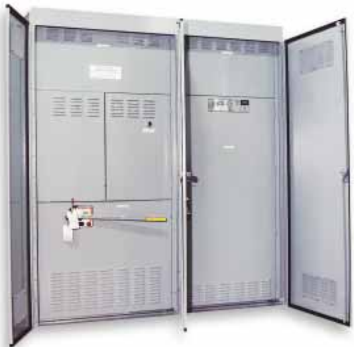
Fig. 18 Transfer switch in an outdoor enclosure.
